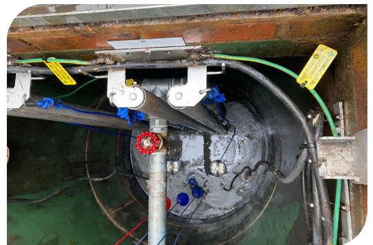
Thames Water SSPS small pumping station including flygt pumps, guide rails and float switches.
