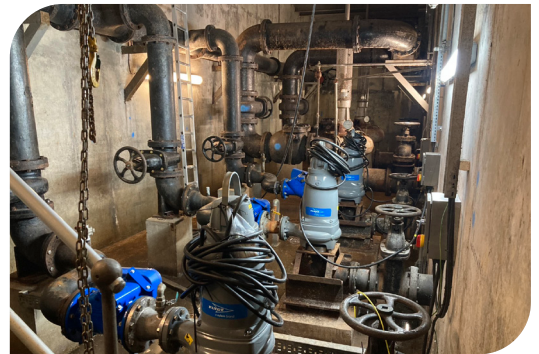
Flygt Concertor dry installed pumps at Llannech Wastewater Pumping Station.
