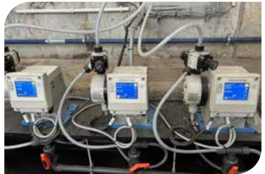
New membrane dosing pumps
