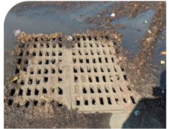
A catch basin grate after a heavy storm at the city's combined sewage pumping station.
