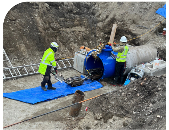
Xylem deploys the PureRobotics platform to inspect the isolated section of the pipeline.
