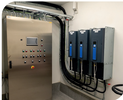
The control cabinet in the main pumping station, including variable frequency drives.
