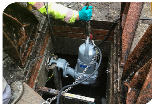
Flygt Concertor at Yorkshire Water's Burnsall car park site.
