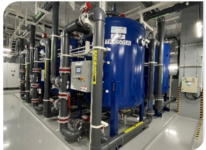
Image 1 Vantage® PTI Multimedia Filtration for pre-treatment.
