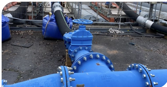
High-capacity bypass pipework diverted flows around the dry well, enabling uninterrupted operation at Irvine Harbour Wastewater Pumping Station.
