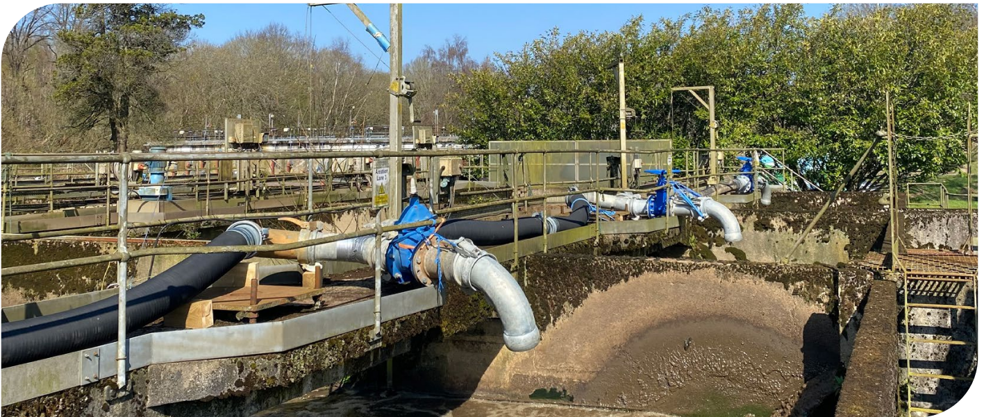
Temporary bypass pumping system maintaining aeration flows during screw pump maintenance.
