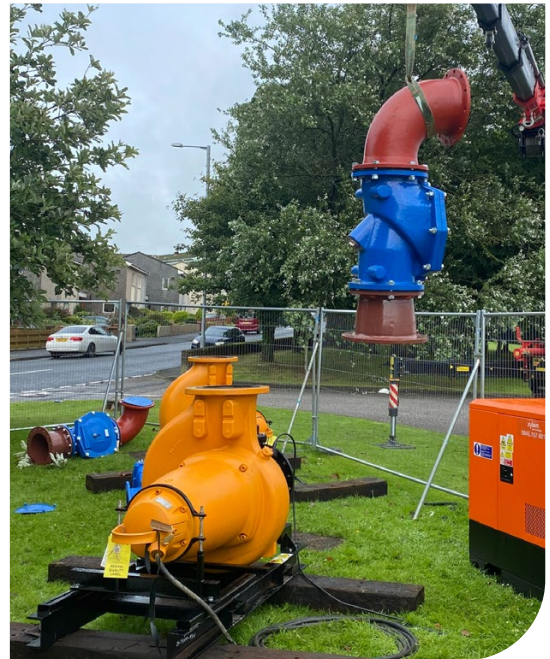
Top: 500 mm discharge pipeline providing high-capacity flow transfer across the temporary bypass network.
