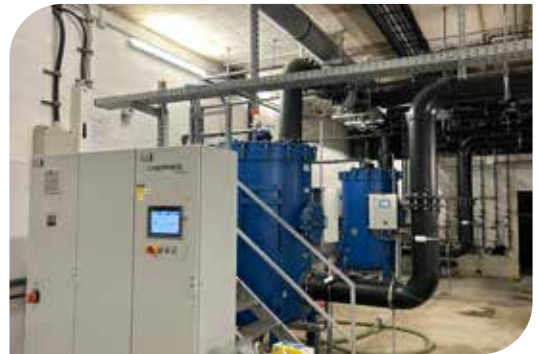
Technical room with new media filters
