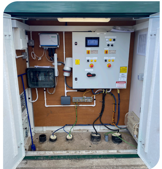
Real-time monitoring and control equipment used to track conditions at one of the pumping stations feeding St Nicholas Sewage Pumping Station.
