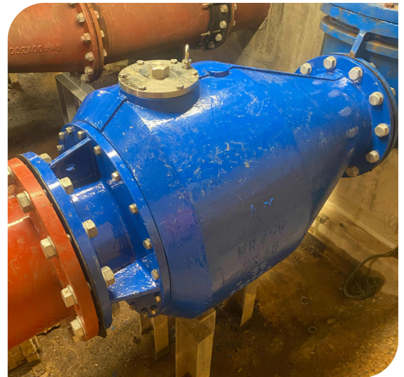
New non-return valve installed at St Nicholas Sewage Pumping Station.
