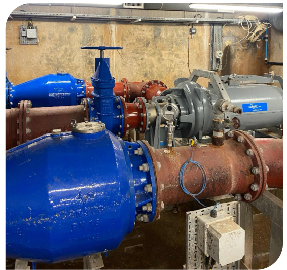
Pumps and associated equipment inside the dry well at St Nicholas Sewage Pumping Station in St Andrews.
