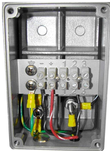
Figure 3-5 Inside the LX Junction Box
