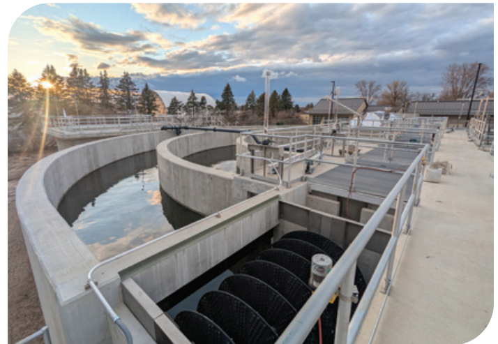
Xylem’s Orbal system in operation with Ox Disc Aerators providing superior mixing efficiency, low energy usage and minimal maintenance.
