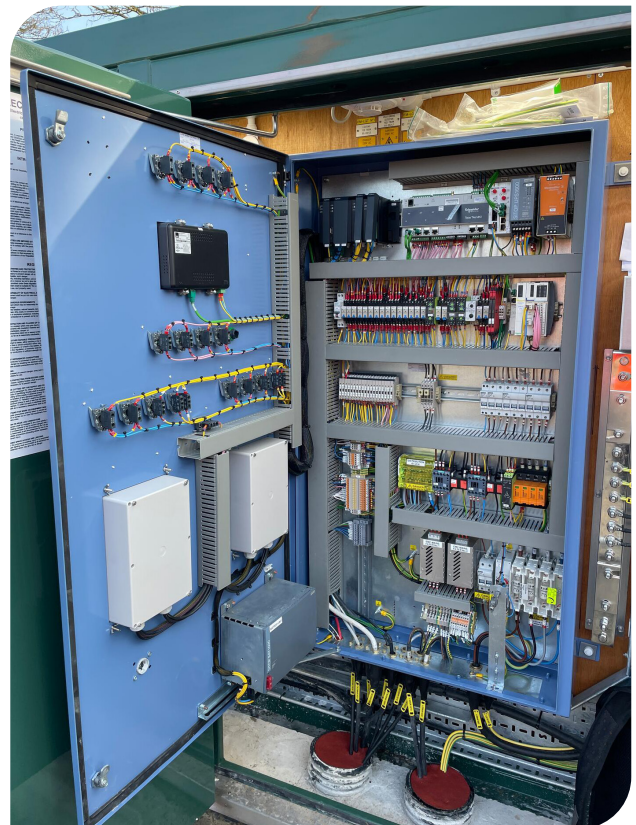
Integrated controls and monitoring on a United Utilities site.
