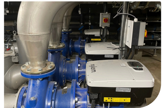
Lowara pumps installed at Doncaster Dome
