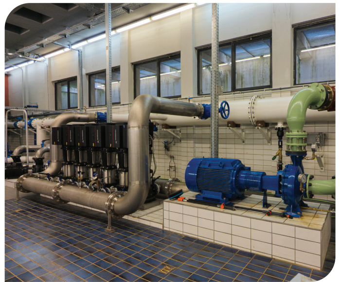
Fig. 3: In the pump station, the treated drinking water is pumped into the distribution network
