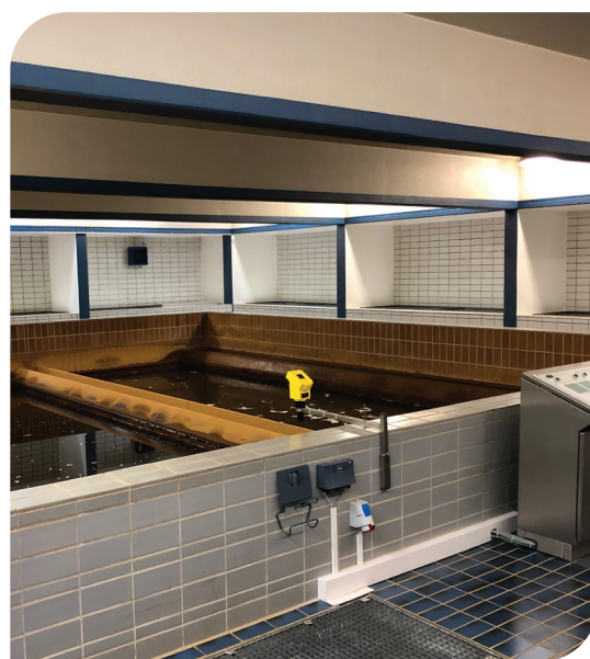
Fig. 1: View of the gravel filter system at the Eutin waterworks
